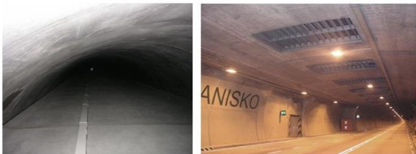
Fig. 4 Ventilation duct and ceiling board of tunnel with flaps for combustion gases exhausting
