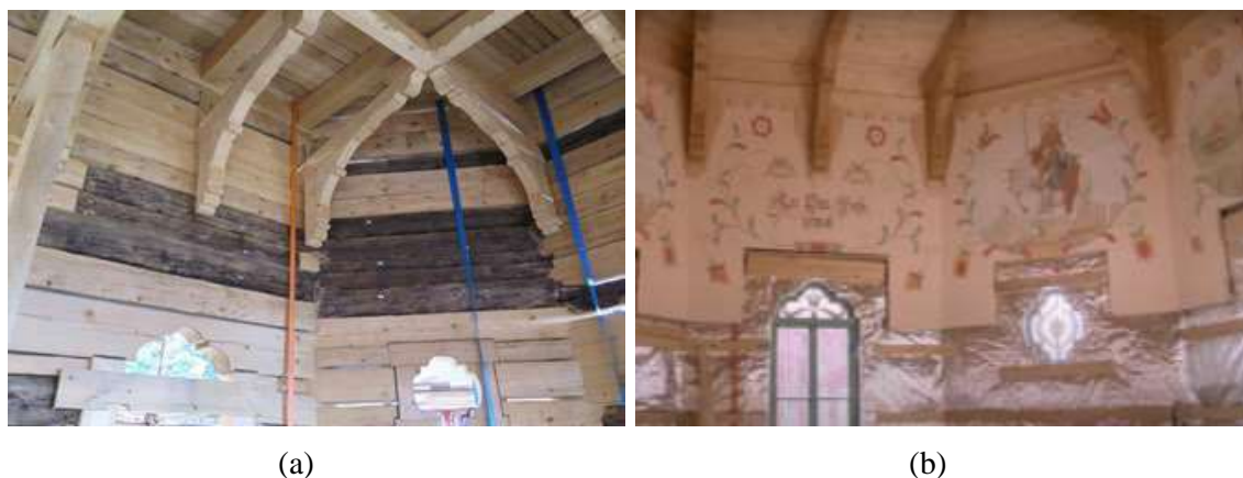
Fig. 2 (a) Log cabin wall with built-in original beams (Novák, 2018); (b) Paintings and frescoes in the new dining room, the vapour barrier is also visible in the lower part (Masák & Partner s.r.o., 2021).
